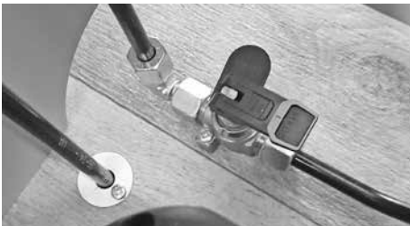
Shut-off valve for the heating system
