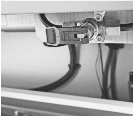
Shut-off valve in the kitchen
